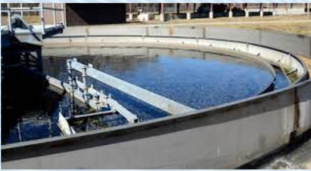
Figure: Biological Aeration Systems and Secondary Clarifier (Rumbaugh, 2023).
