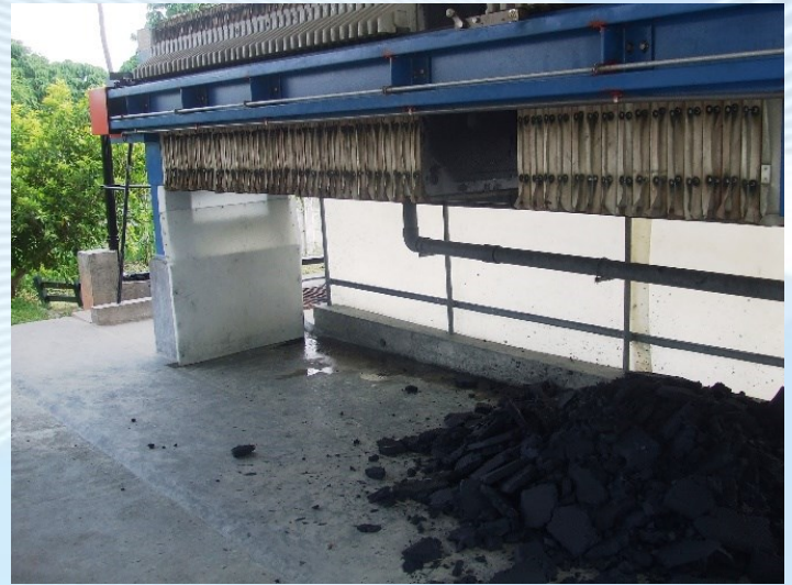
Figure: Separated Sludge Slurry Filter Pressed
