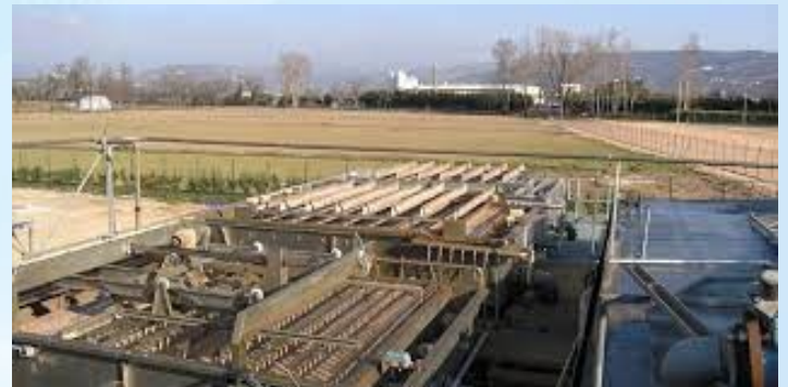
Figure: Chemical treatment Dissolved Air Flotation system (Fluence Corporation 7135 Madison Ave. West Golden Valley, 2024).
